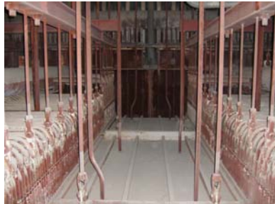
"The Attic" with 2500mm between hanging pipes
