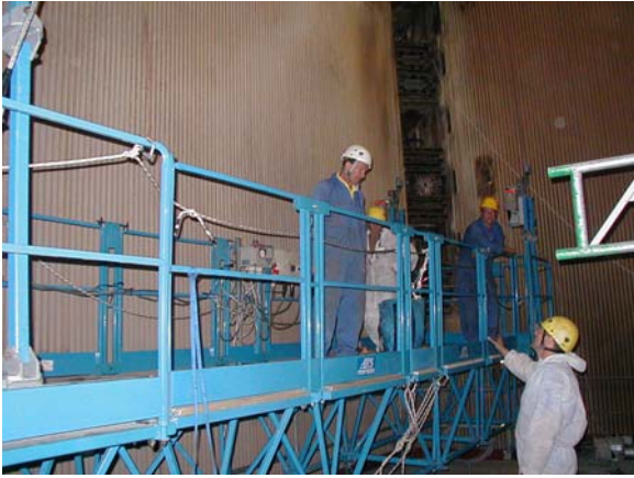
The "Boiler Chamber" with Steel Truss Frame platform completed and undergoing examination.
