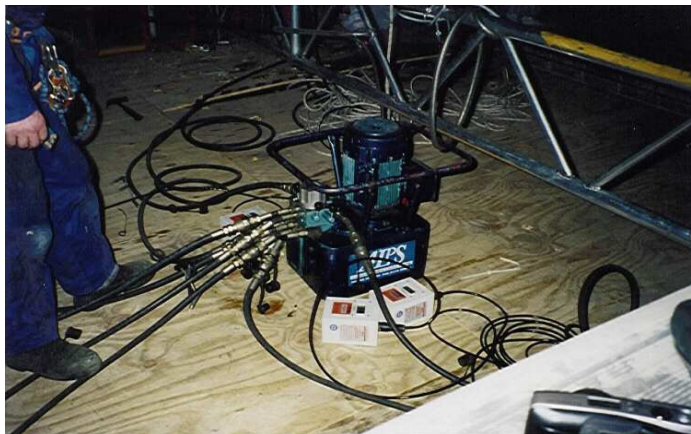
4 way power pack, control valves & digital load indicators
