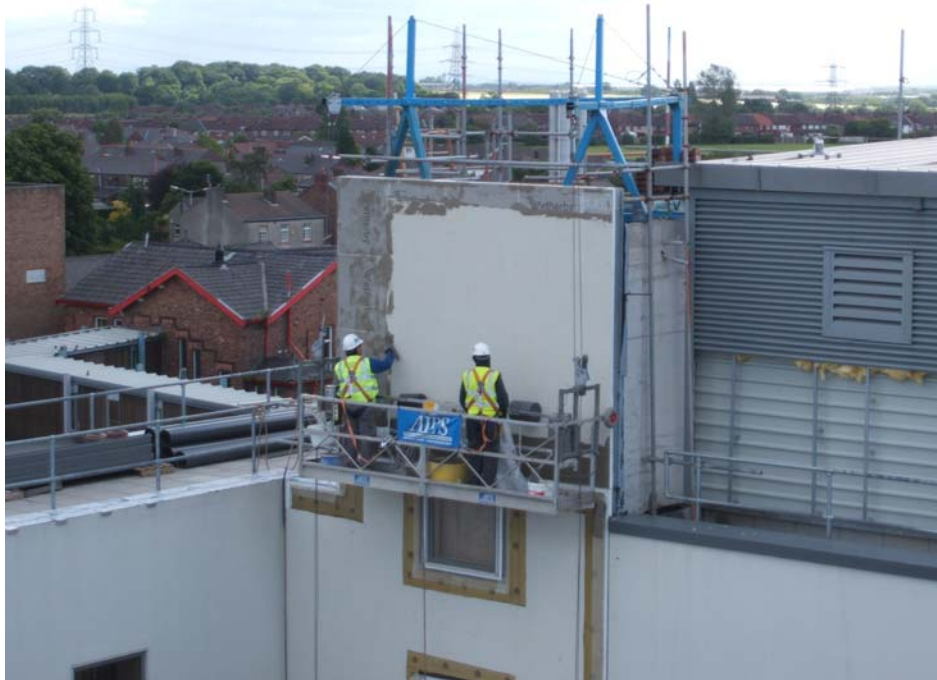
3M platform suspended from portable telescopic roof beams
